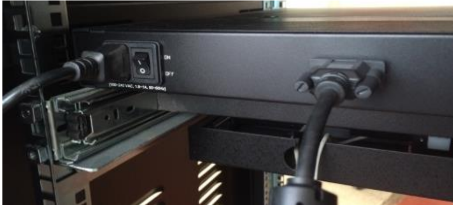
Figure 5 Power and VGA cables
