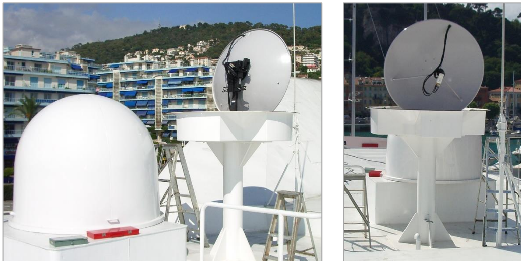
Figure 72. Typical ADE Installation
