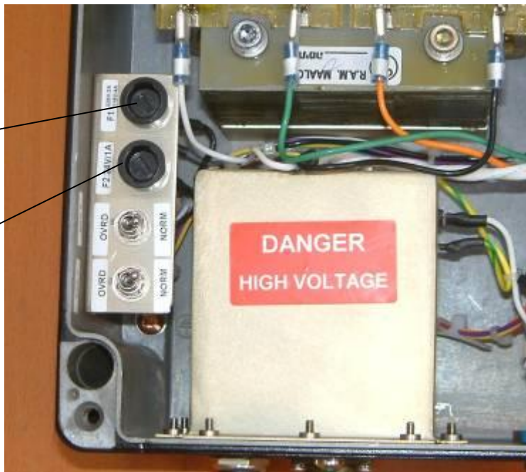
Figure 9-1. SDU Internal View
