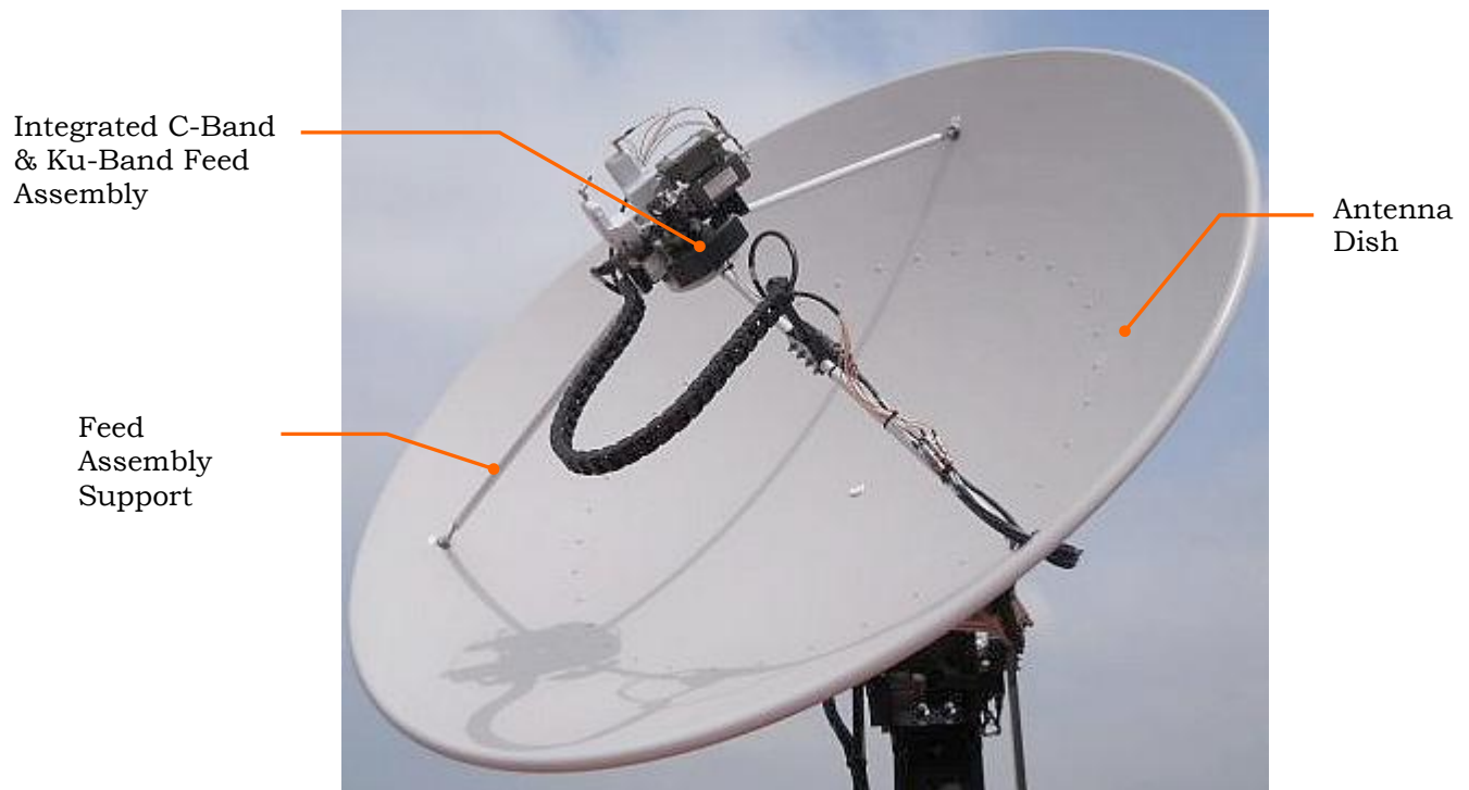
Figure 2-4: Feed General View
