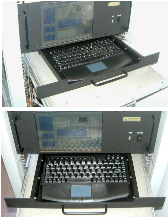
Figure 10-1: Typical BDE Rack Installation
